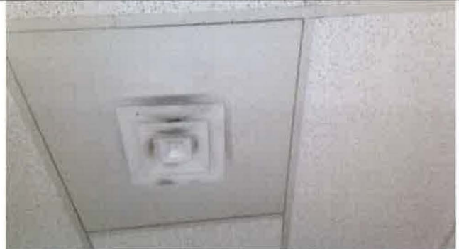
Dirty HVAC supply diffuser in Room 403
