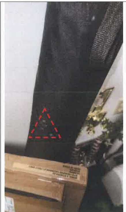
Moldy equipment case in storage room
