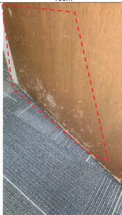
Moldy door in storage room
