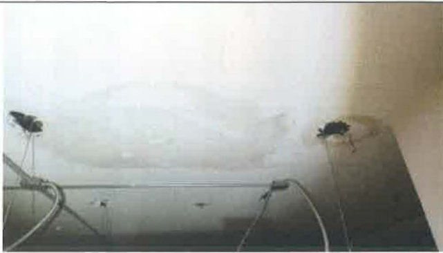
Water damage noted to drywall ceiling in multiple locations
