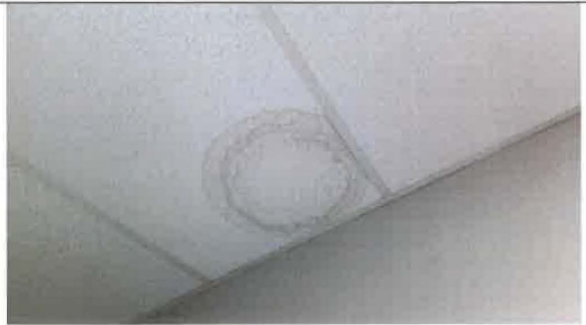
Water damage was noted to drop ceiling tile in multiple locations
