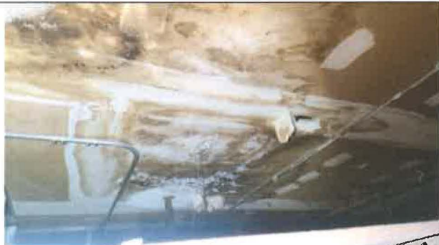
Water damage noted to drywall ceiling in Room 418
